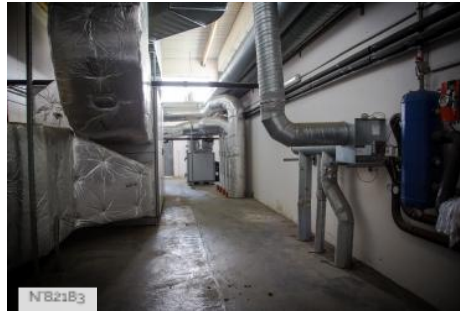
City of Evry-Courcouronnes - Lake sports complex - Boiler room
