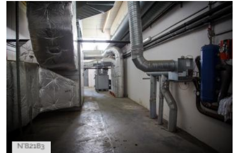
City of Evry-Courcouronnes - Lake sports complex - Boiler room
