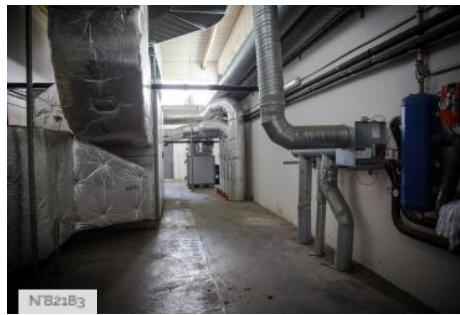
N'82183 City of Evry-Courcouronnes - Lake sports complex - Boiler room
