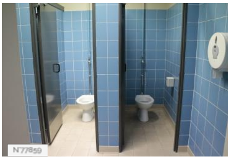
Aubervilliers Jean Macé School - 1st floor sanitary
