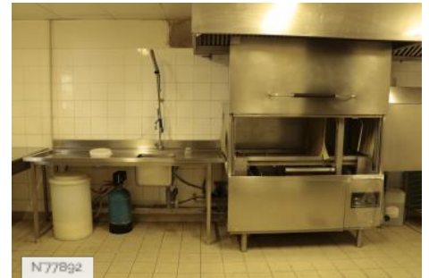
Aubervilliers School Jean Macé - Kitchen
